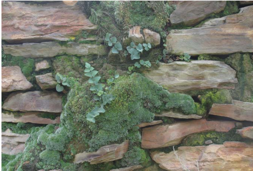
Figure 13. Moss-covered plastered remains on the wall of the dwelling. 84
